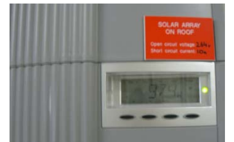
Top & Above: Solar energy inverter
