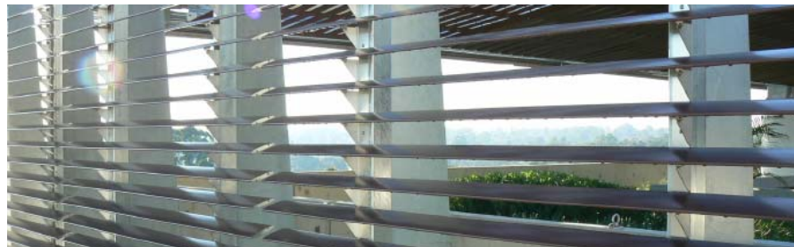
Top Left: Western façade – Louvers. Top Right: Internal Louvre controls. Above: Louvers
