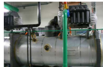
Top & Above: Chillers
