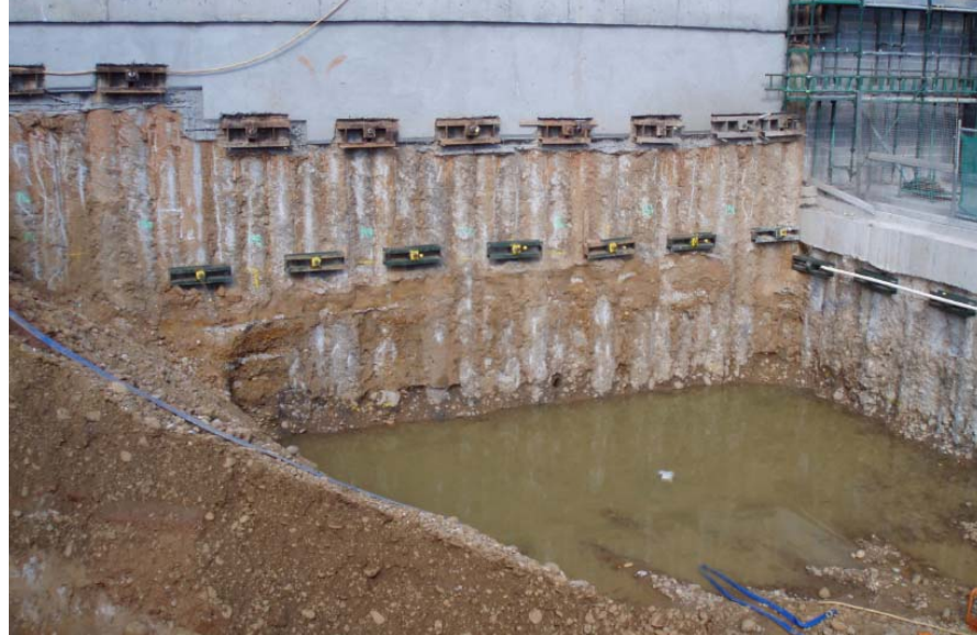
Above: Water Issues during Excavation
